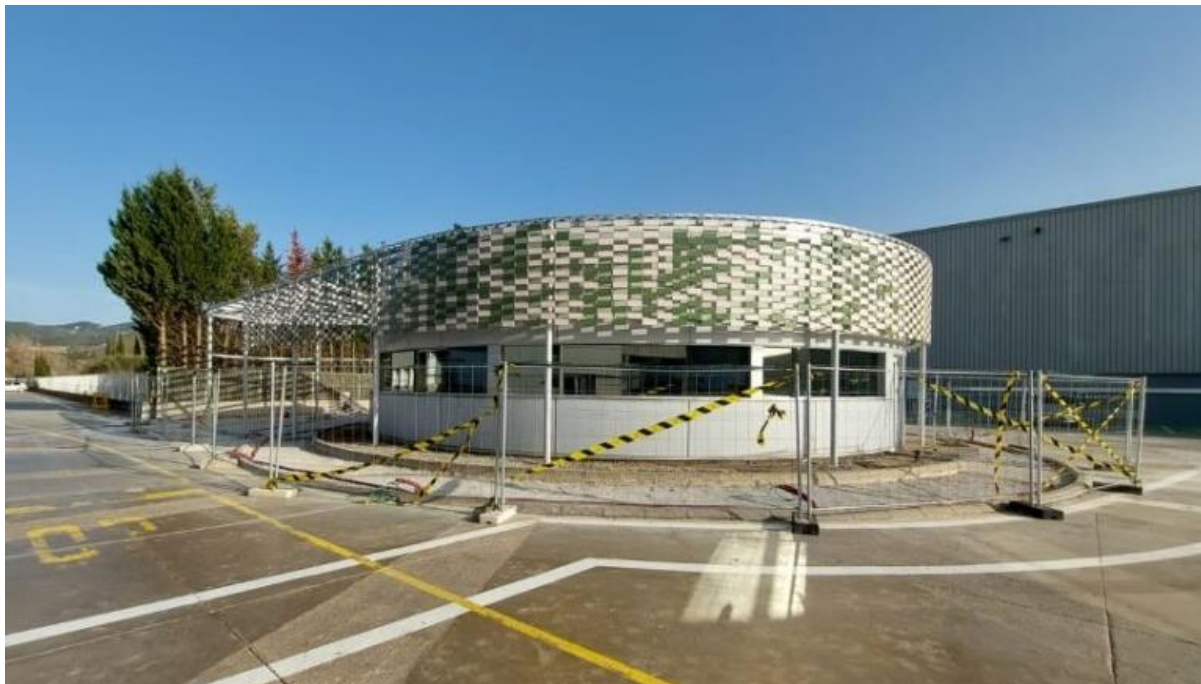
Figure 27 Control building in Sant Sadurn d'Anoia with partly installed integrated PV in an interwoven steel wire mesh – Living lab no. 24
